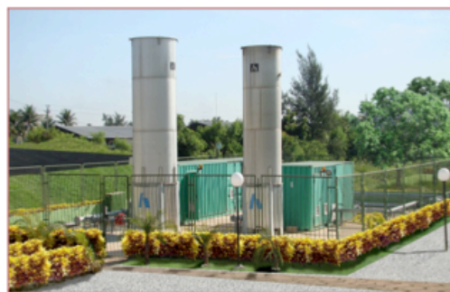
3. Torch system for flaring biogas.
