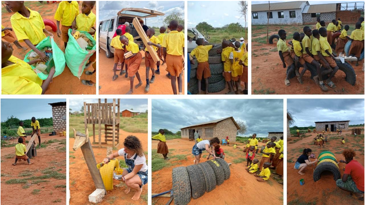
Figure 7: Photos of the construction of the playground: collection of plastic materials and cleaning of the area, unloading and preparation of materials (cutting and preservative treatments), assembly of playground equipment, and painting.
