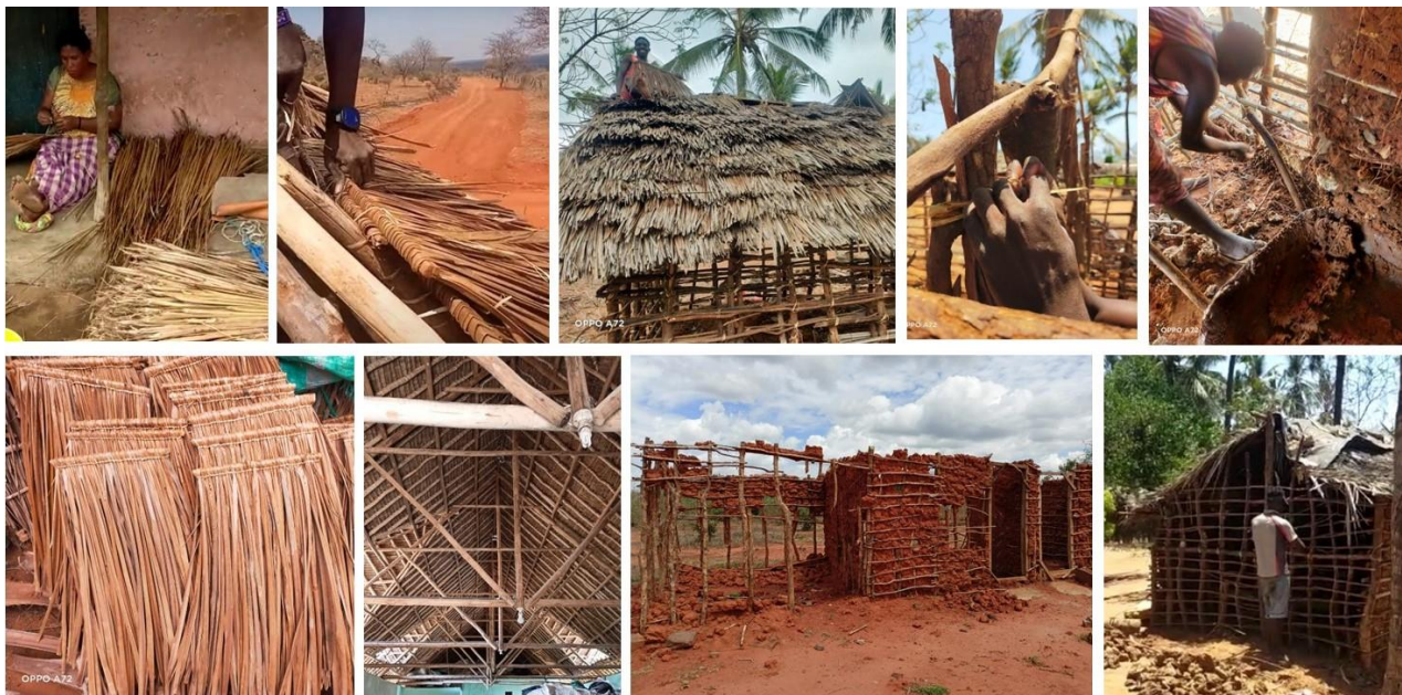
Figure 2: Building system based on raw earth, timber, and makuti roofs. Construction steps and installation of makuti and construction process of a typical housing.
