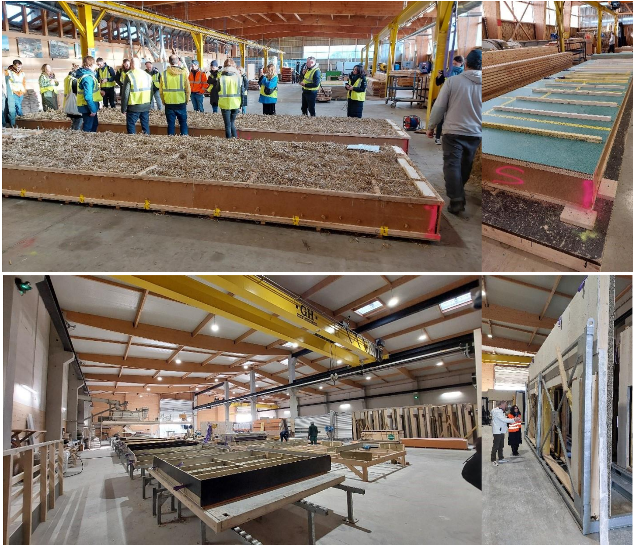
Figure 17: Showing straw based (above) and hemp based (below) biobased modular wall panel manufacturing facilities. Chênelet (straw) & Wall'Up Prefa (hemp) Northern France [Source Authors].
