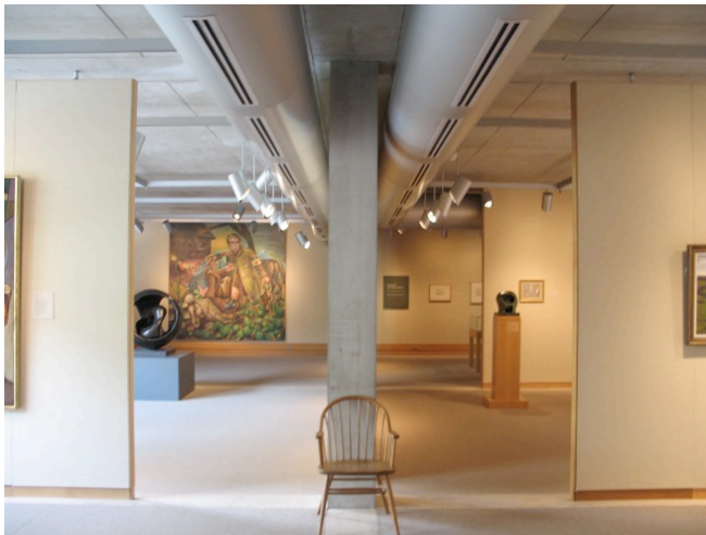
Figure 13: Exposed integrated outtake ventilation pipes.
