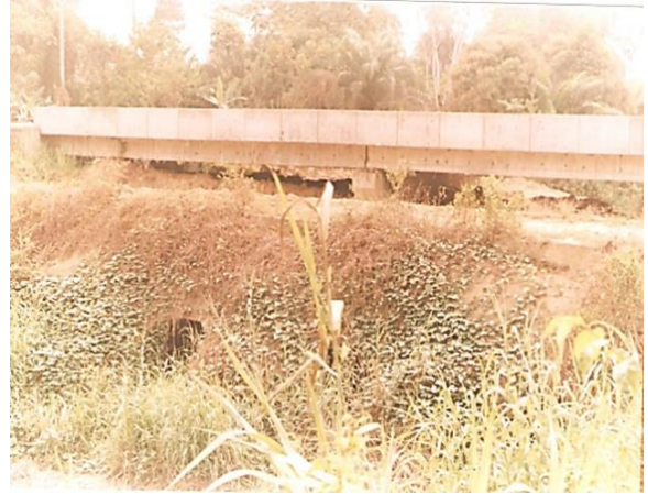
Figure 10: Unhealthy Interaction between Recent Road Network and Existing Drainage Culvert (D-02 at Agbura Axis) (Source: NPFC 2013).
