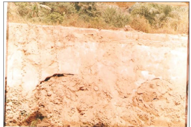
Figure 11: Completely Silted/Blocked Armco Culvert on Drain D-02 Alignment at Agbura (Source: NPFC 2013).
